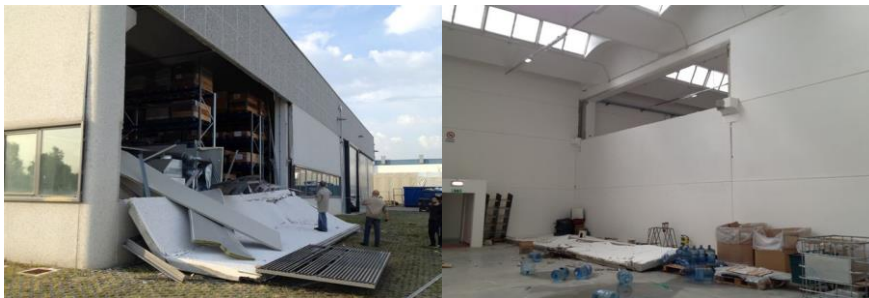
Fig. 3. Emilia 2012: panel failures – peripheral cladding and internal partition walls.
