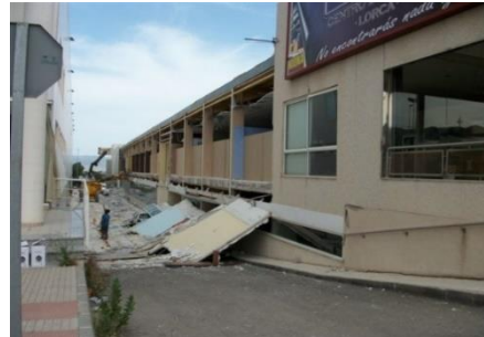
Fig. 2. Lorca 2011: structure OK, panels KO.
