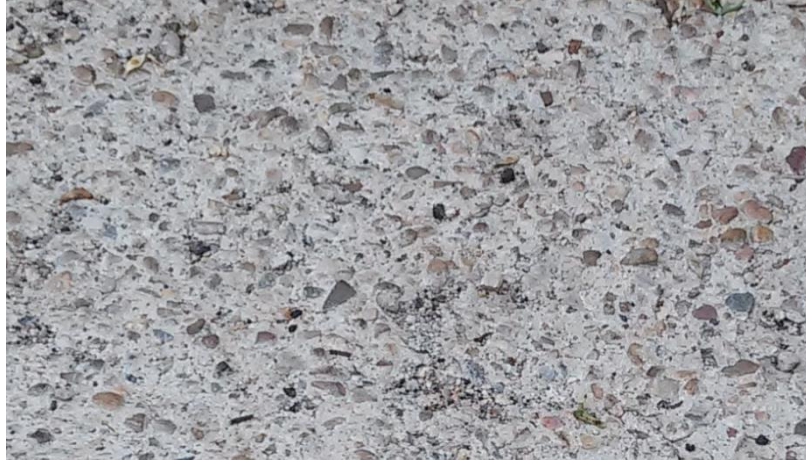
Fig 2: Deteriorated concrete surface at intersections
