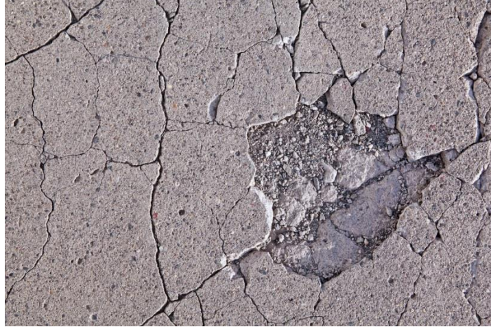
Fig 1: Deteriorated concrete surface due to aggregate expansion
