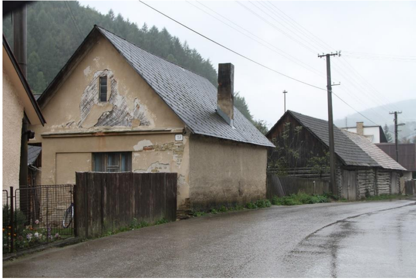
Fig. 1. An old earthen building in the White Carpathians, Slovakia. Without maintenance the buildings rapidly decay. (Photo: U. Herbig)
