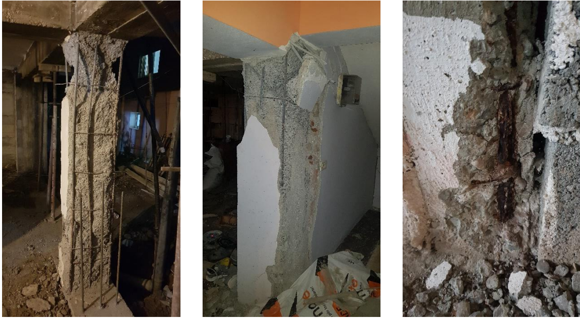
Figure 3. Damages of residential buildings with flexible structural system in IV zone of Durrës
