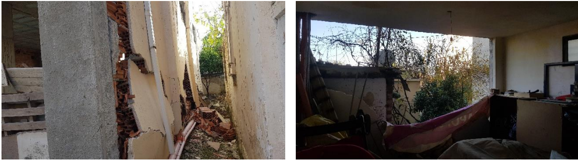
Figure 4. Failure of infill walls of residential structures.
