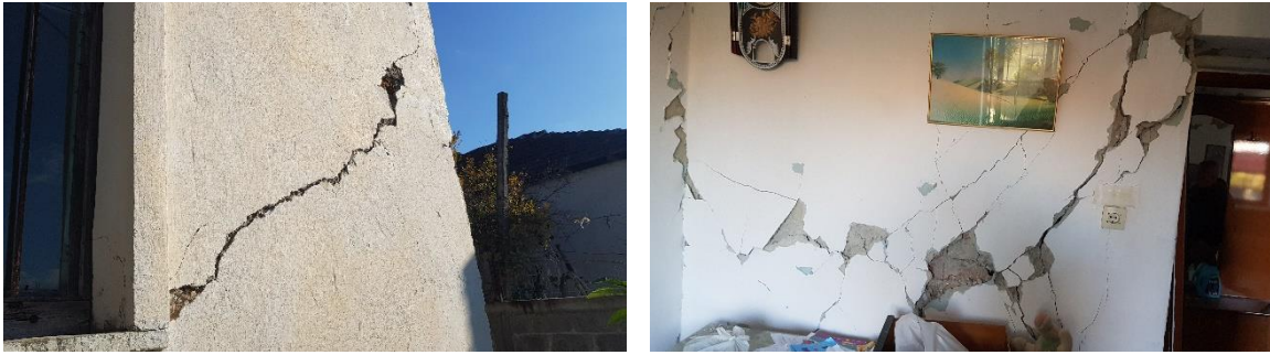
Figure 2. Damages of residential buildings with masonry walls structural system
