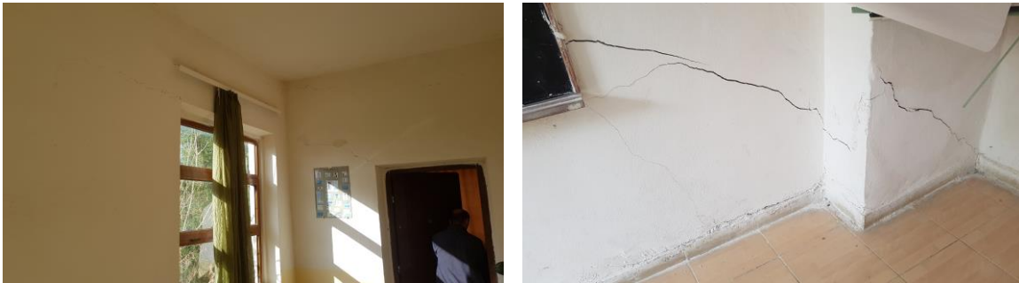
Figure 1. Damages to the school of Karbunare and Hysgjokaj of Lushnja
