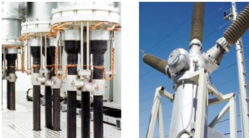
Fig.2. Cable terminators and Air-Gas Bushings
