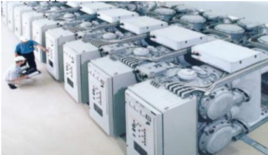
Fig.3. Control and monitoring
